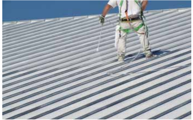
ABOVE ▲ In addition to the safety of the students and neighbors below, the personal safety of the crew was important. Ruff and his team wore Spider construction harnesses with D-ring positioning using rope grabs and 5/8" (1.59cm) rope, to remain safe and comfortable when working on the steeply pitched roof. They also wore respirators and fresh air blast helmets with peel-away shields.
